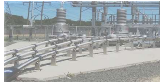
110 kV HTS cable Novel technology
