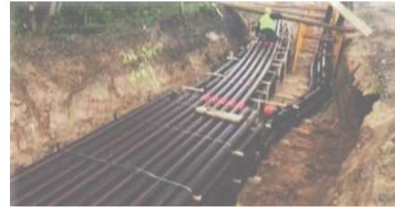
Multiple 110 kV XLPE cable systems 5 systems & routes
