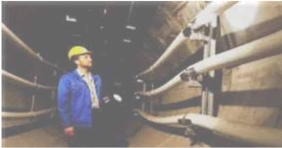
400 kV XLPE cable system E.g. tunnel solution, as in Berlin, London
